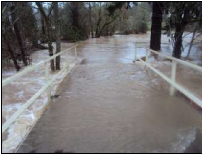
Bridge over Mill Creek is under water.
